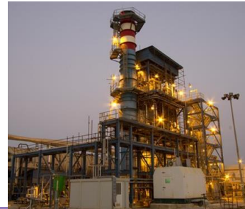
STEAM THERMAL POWER PLANT WATER TUBE BOILERS
